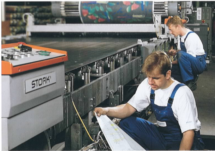
Installation of the standard "Individual drive" package means that the existing mechanical drive is removed.
